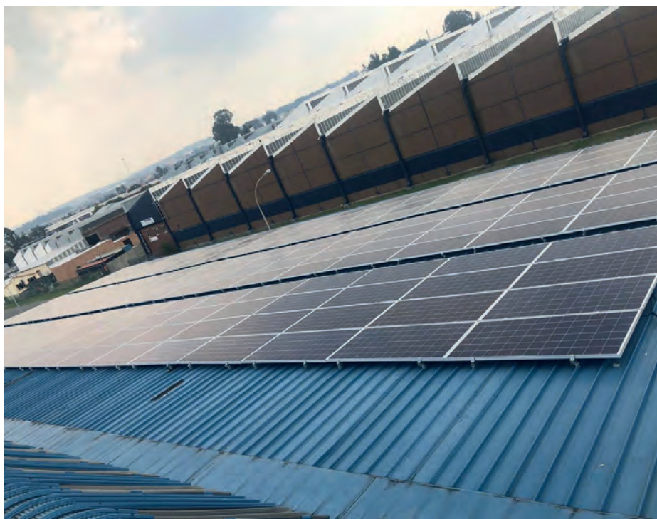
Hyundai's recent solar PV installation at its PDC in Gauteng.
