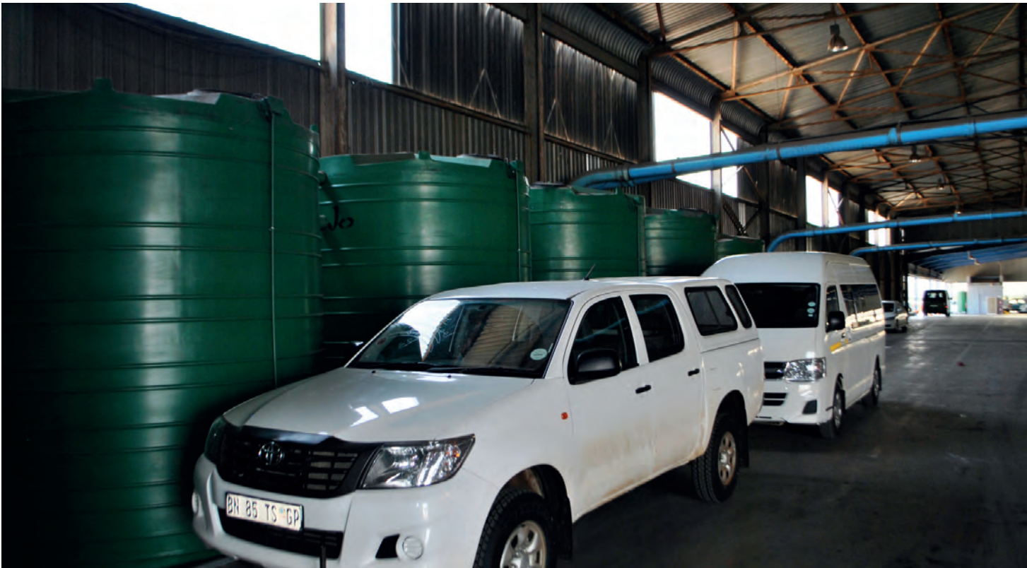
Rainwater harvesting system at our Jet Park car rental depot.
